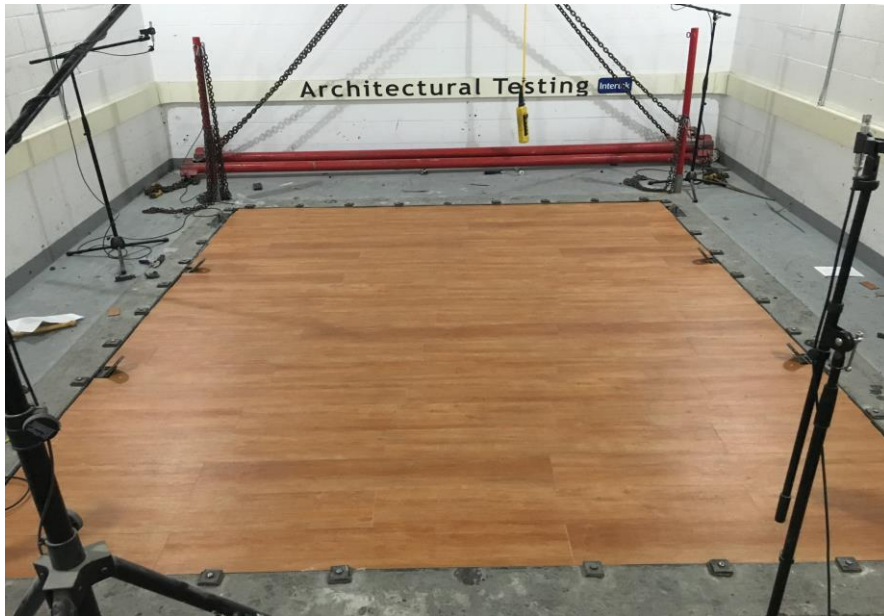
Source Room View of Test Specimen Installation
